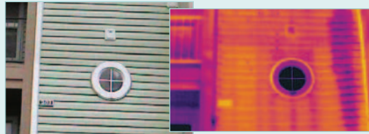
The thermogram of the apartment building shows the path of a serious leak, completely hidden within the wall, from a washing machine on the third floor
