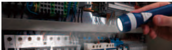
Erroneous circuit-breaker activation
