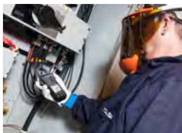
Analyze Power-related Issues
