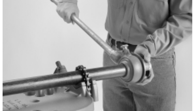
Figure 3 – Sliding Threader On Pipe
