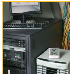
Alerts low Humidity levels in Computer rooms to help prevent electrostatic conditions.
